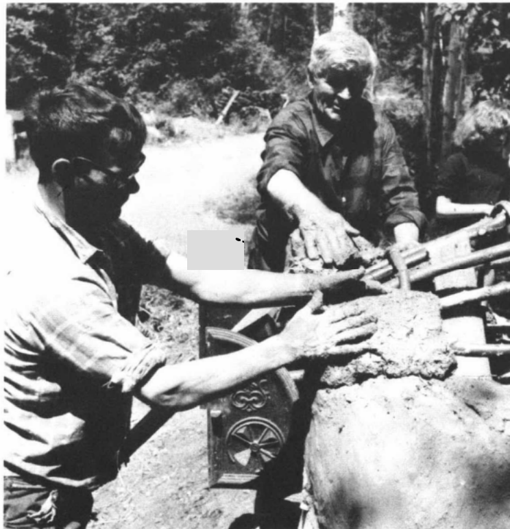
The clay blocks are laid around the arch of the doors Lise and Jean-François Blanchette Collection
